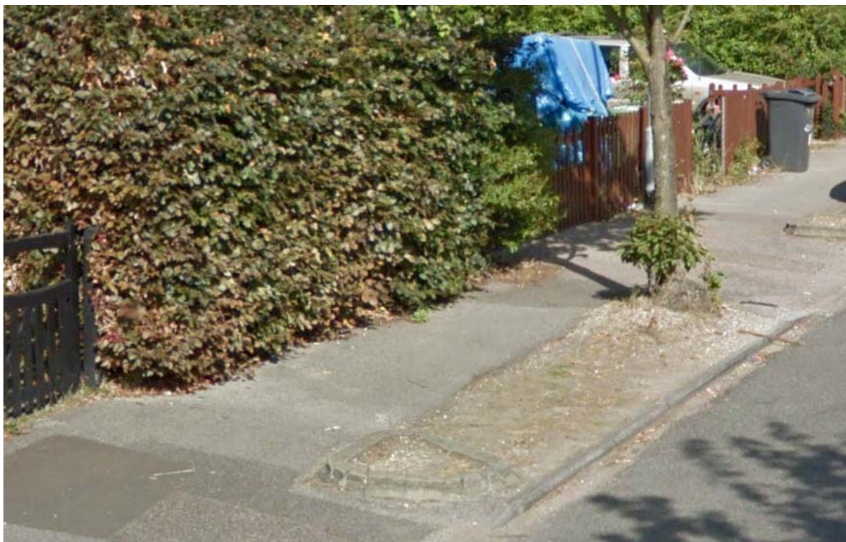
Photo of Existing Location: (One of the existing planters which is in a poor condition)
